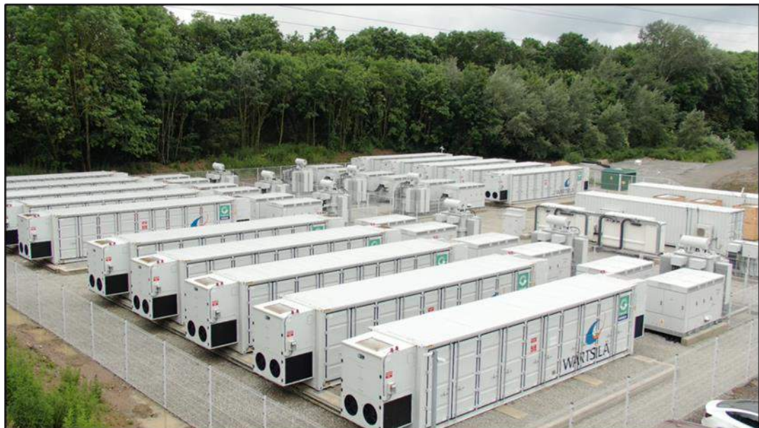
Figure 2-4: Example BESS facility
