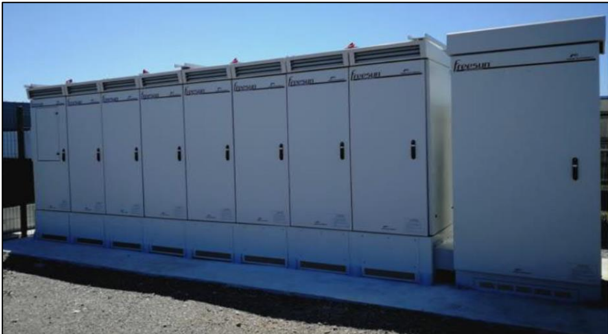
Plate 2.4 Typical outdoor centralised inverter
