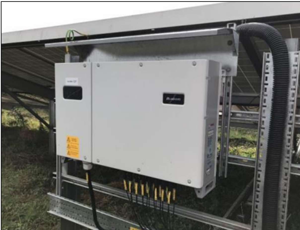
Plate 2.3 Typical string inverter
